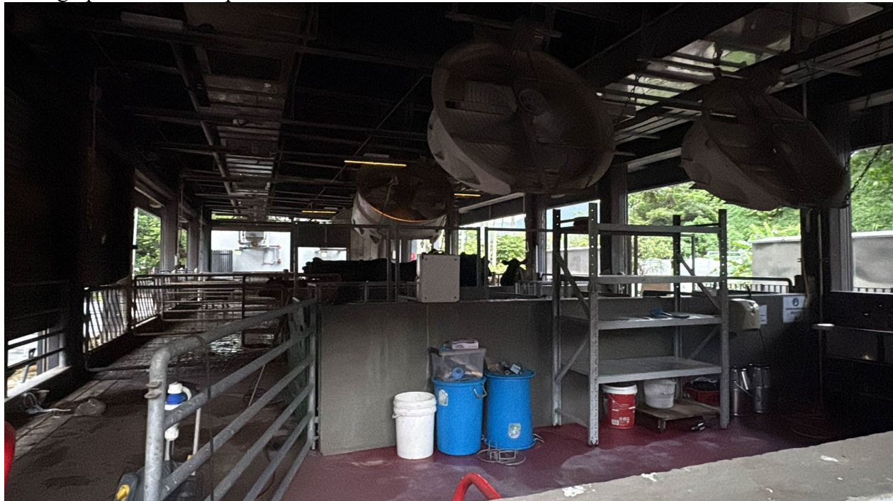
Photograph for defect reported on 07/09/2025
